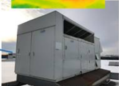
AAON HEATING-COOLING-VENTILATING UNIT
